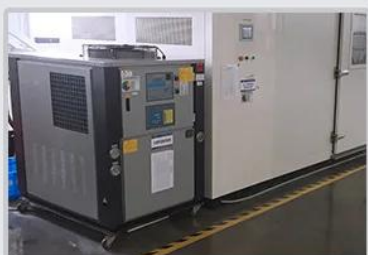
Aging Test Room
