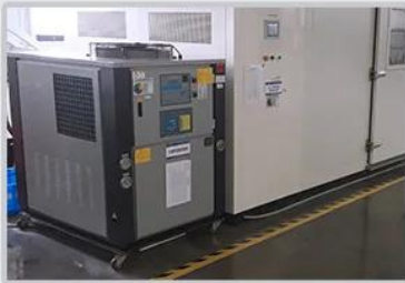
Aging Test Room
