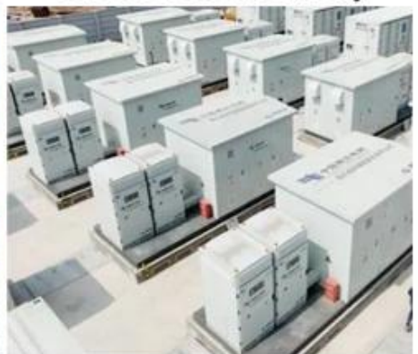
Utility grid/Ups systems/
