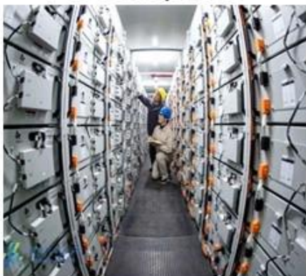
Industrial energy storage
