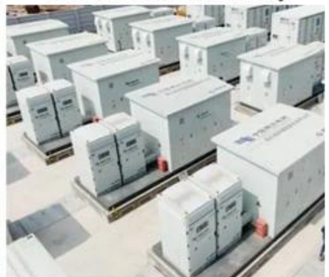
Utility grid/Ups systems/
