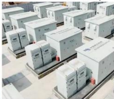
Utility grid/Ups systems/
