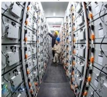
Industrial energy storage
