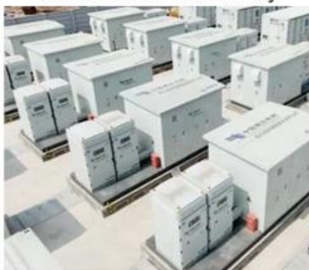
Utility grid/Ups systems/
